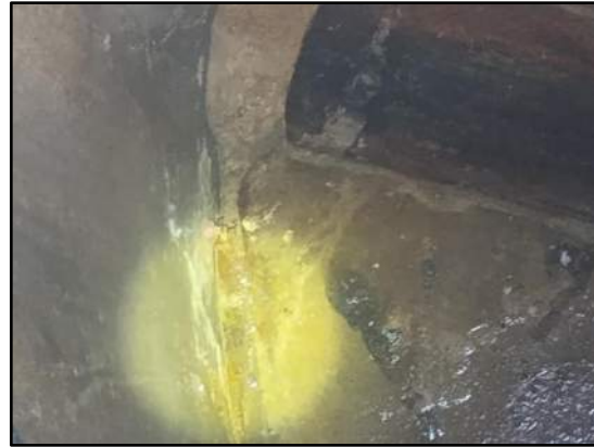
MH 25-010, infiltration from cracks in base
