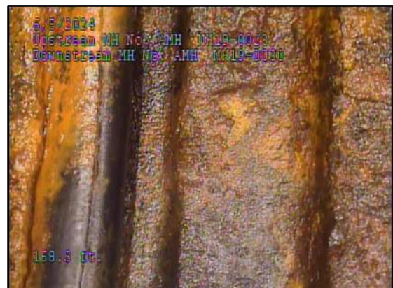
MH 19-0028 to MH 19-0030, large joint separation, gasket visible
