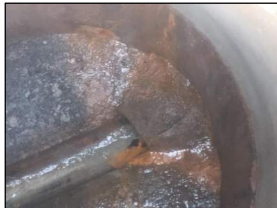
MH 19-0023, infiltration at North connection
