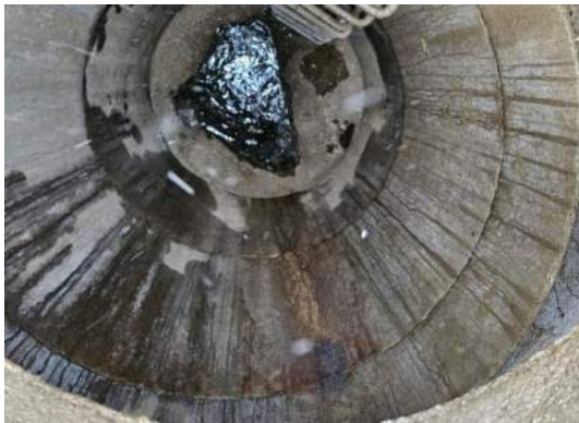
I&I seeping through joints
