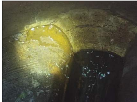
MH 25-003, infiltration at influent connection
