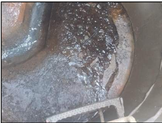
MH 19-0030, infiltration and eroding shelf
