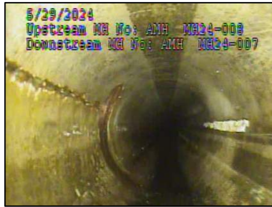
MH 24-008 to MH 24-007, longitudinal fracture and infiltration runner at tap connection
