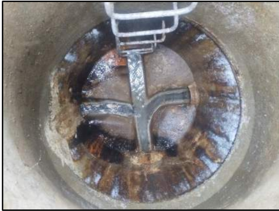
MH 25-004, infiltration and cracks in base
