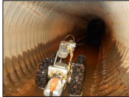
Typical CCTV Camera in Pipe
