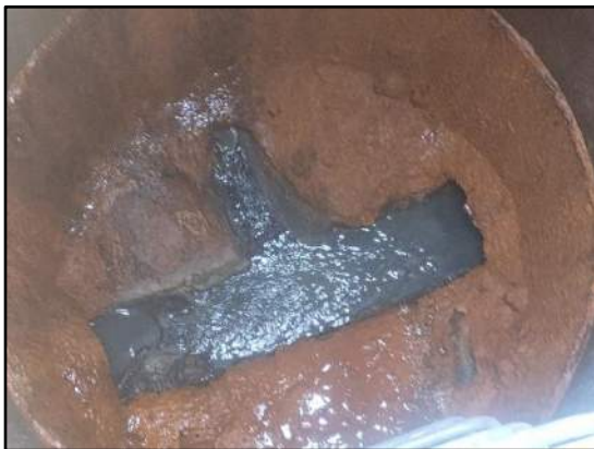
MH 19-0021, infiltration at cone-base joint
