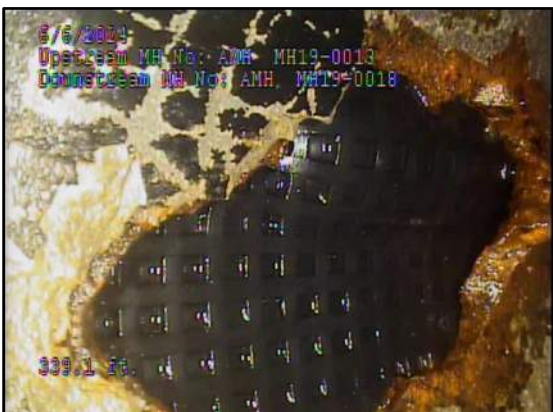
MH 19-0013 to MH 19-0018, defective repair patch with I&I coming through
