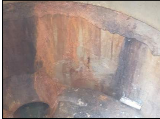
MH 19-0028, infiltration and offset
