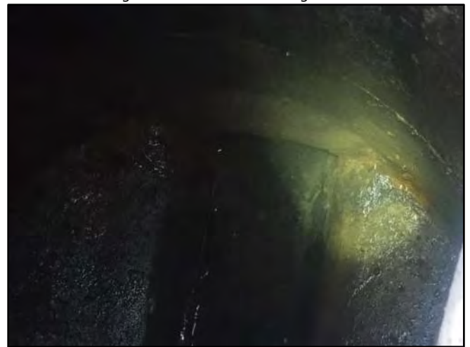
Image 6 – Missing Concrete and I&O dripper
