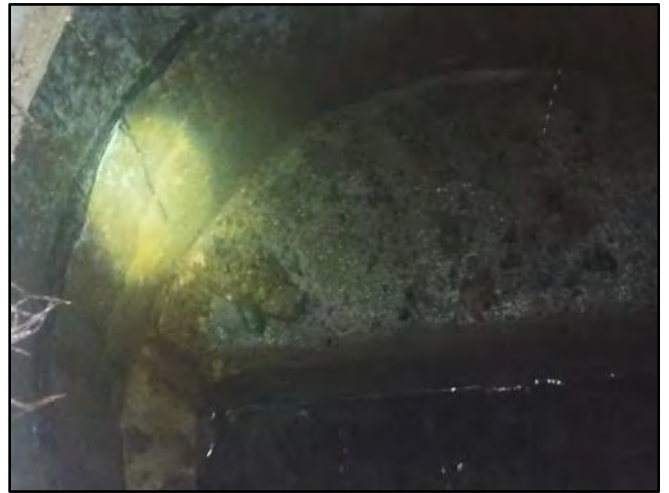
Image 4 – Large Crack in Base pt. 2
