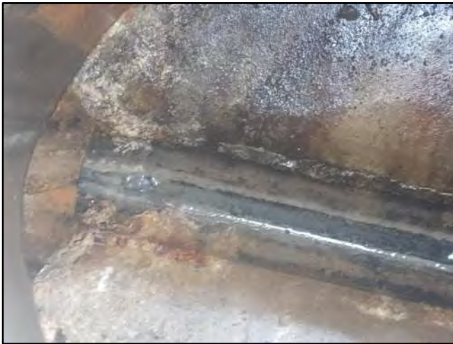
Image 3 – Dripper along East side of South Connection
