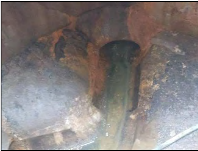
Image 5 – I&I along South Effluent
