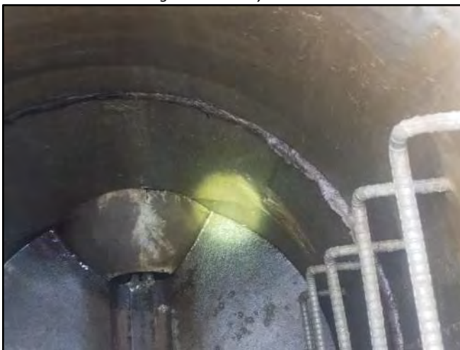
Image 5 – I&I runner along West Side, Crack
