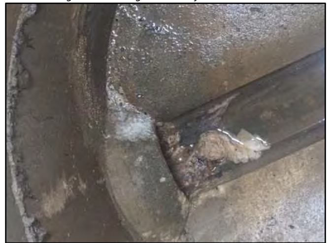
Image 6 – North Effluent Connection
