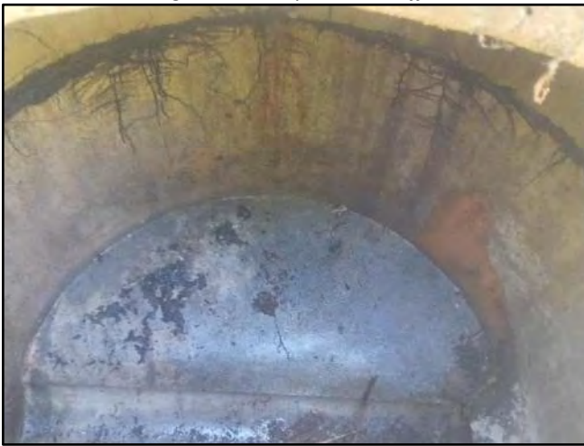
Image 5 – Root Intrusion at Cone/Base Joint
