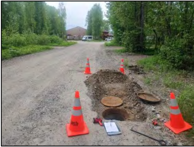
Image 1 – MH facing South on I St
