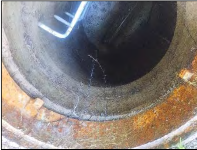
Image 3 – Roots at Structure's Joints
