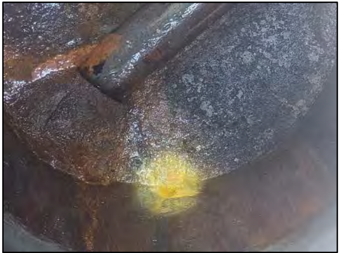
Image 4 – Missing Concrete and Dripper
