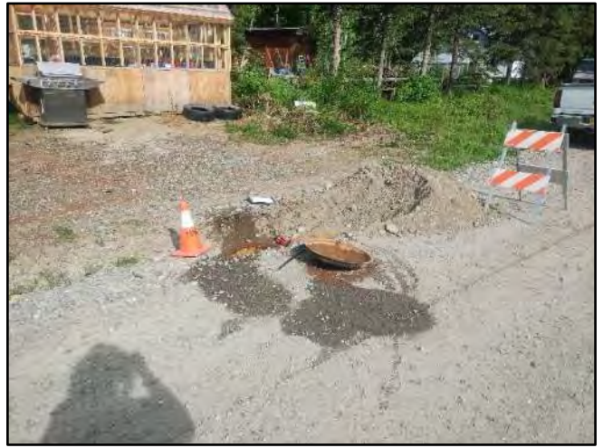
Image 2 – MH facing towards Green House
