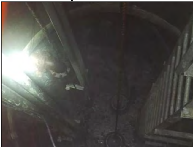
Image 5 – North Effluent Pump Connection
