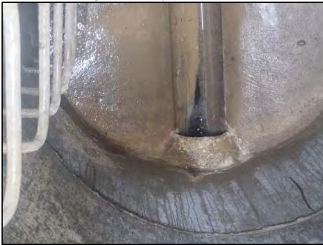
Image 5 – I&I Dripper to the West of North Connection
