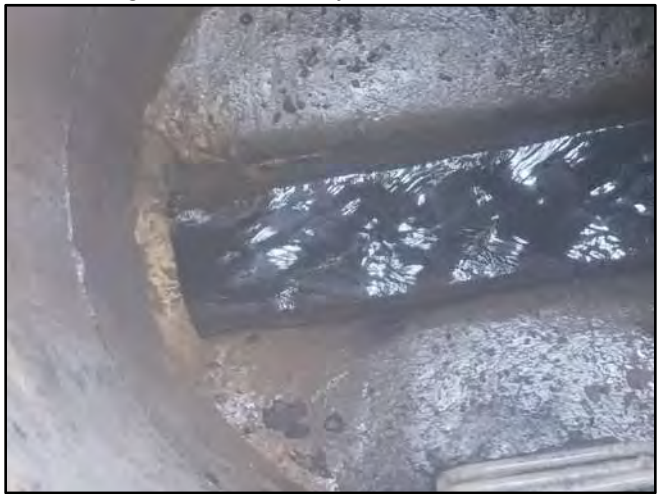
Image 6 – North Effluent Connection
