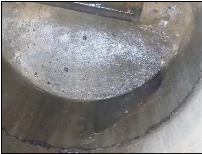
Image 3 – Crack along West side of base
