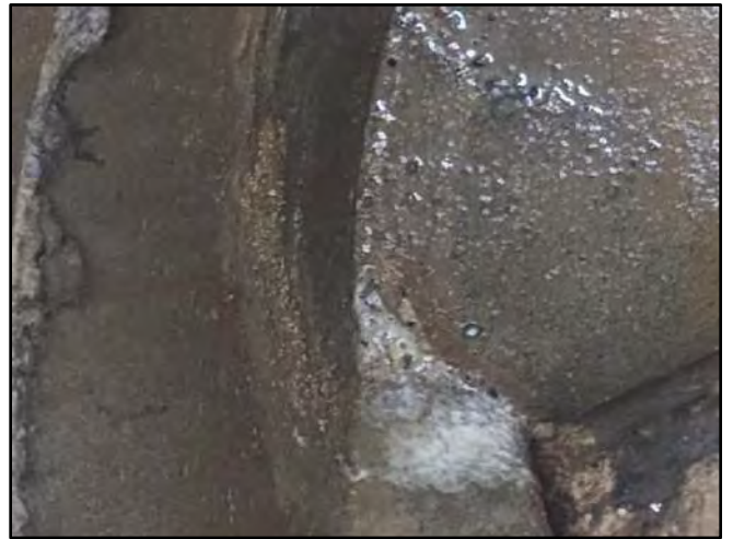
Image 4 – I&I along East side of North Connection
