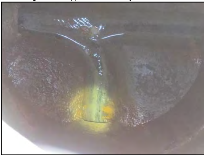
Image 5 – I&I Drippers and South Influent Connection
