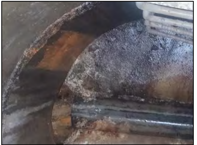
Image 4 – Flowlines along SW Base
