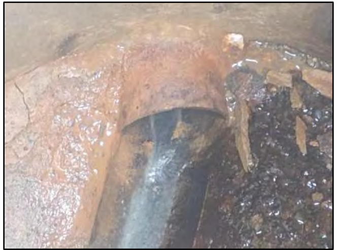
Image 4 – Influent Pipe Connection
