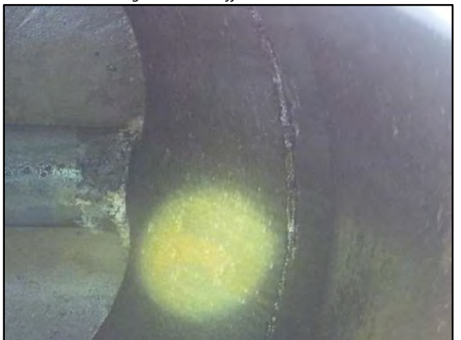
Image 6 – Flowlines from Cone/Base Joint
