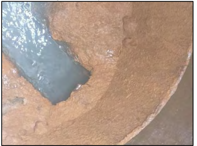
Image 6 – North Effluent Connection
