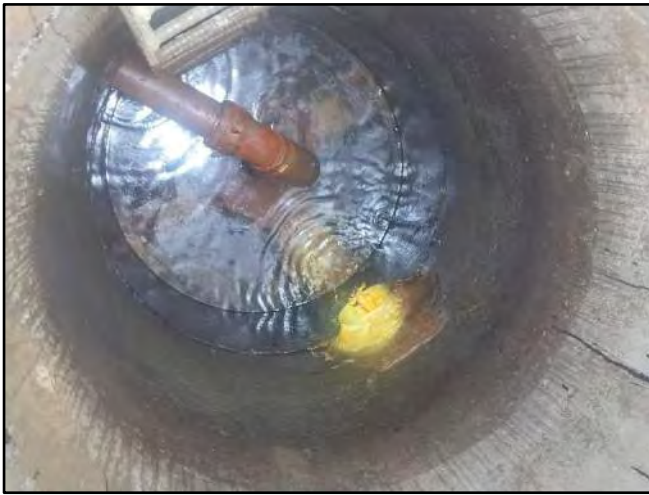
Image 3 – North Decommissioned Connection
