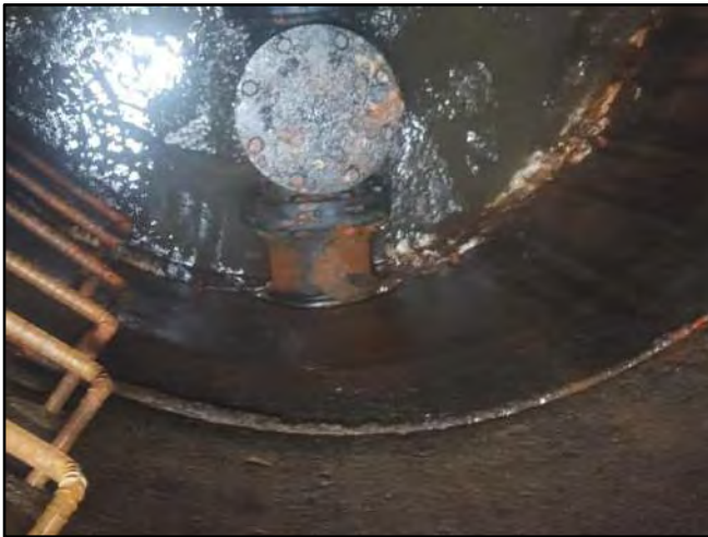
Image 3 – South Connection with Large Cracks and Heavy I&I
