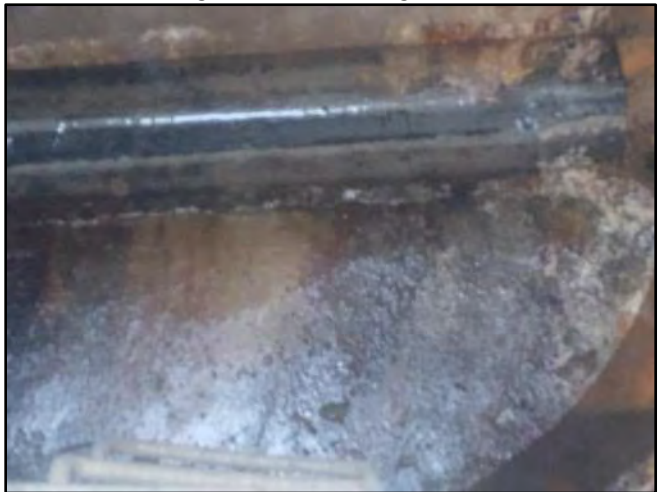
Image 6 – Moisture along West Shelf
