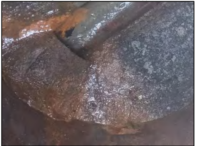
Image 6 – North Effluent Connection
