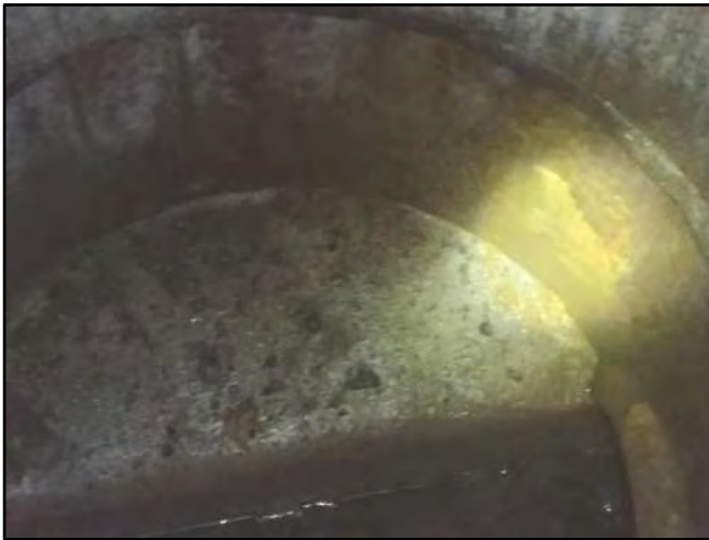
Image 3 – Large crack in Base
