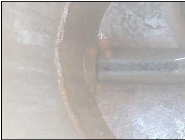
Image 3 – I&I Drippers above East Influent Connection
