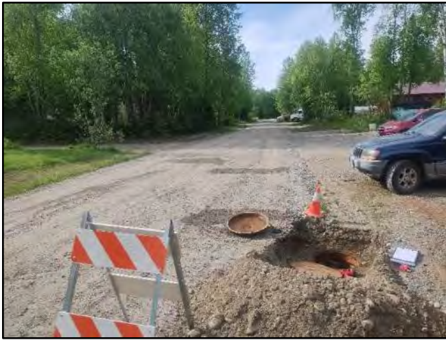
Image 1 – MH facing South on I St
