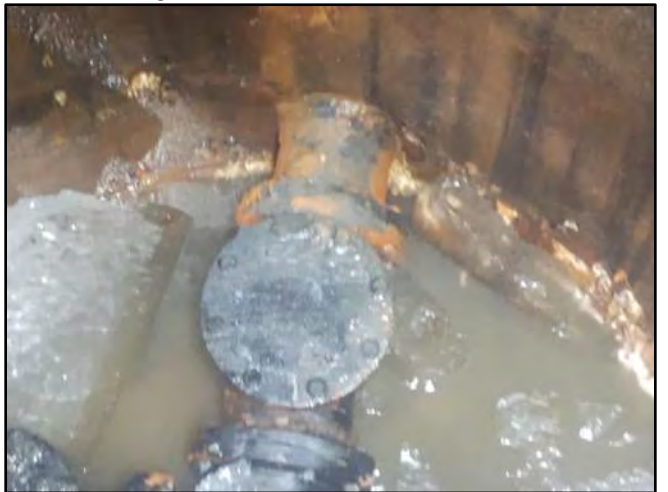
Image 6 – West Connection, Large Cracks
