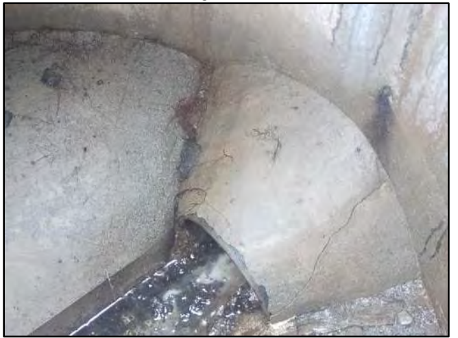
Image 6 – North Effluent Connection
