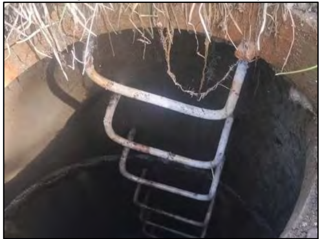
Image 6 – Root Intrusion along top of Cone
