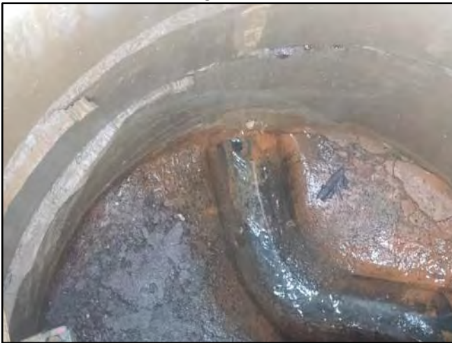
Image 5 – Effluent Pipe Connection
