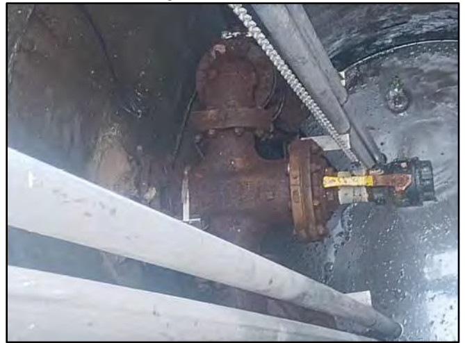
Image 6 – North Effluent Pump Connection
