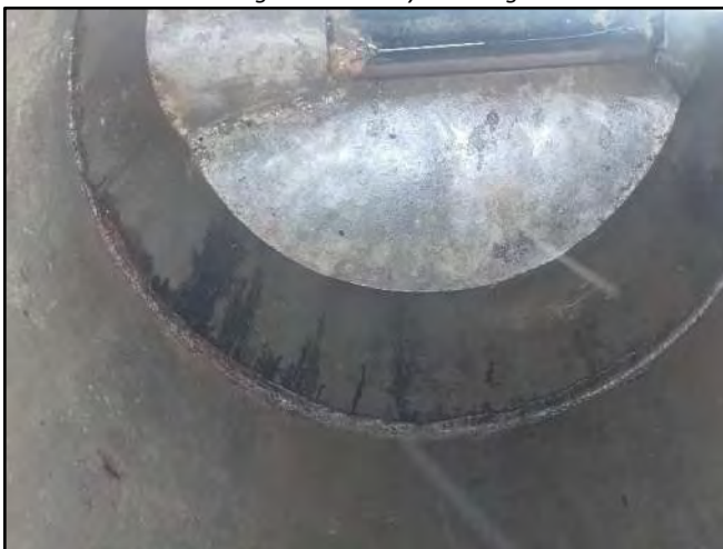
Image 5 – I&I flowlines along West Side
