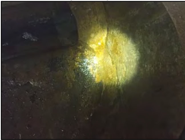
Image 5 – Northeast Influent Connection and Crack
