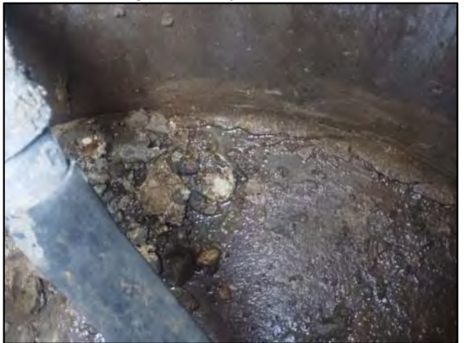
Image 6 – Debris and Moisture along Base's Shelf
