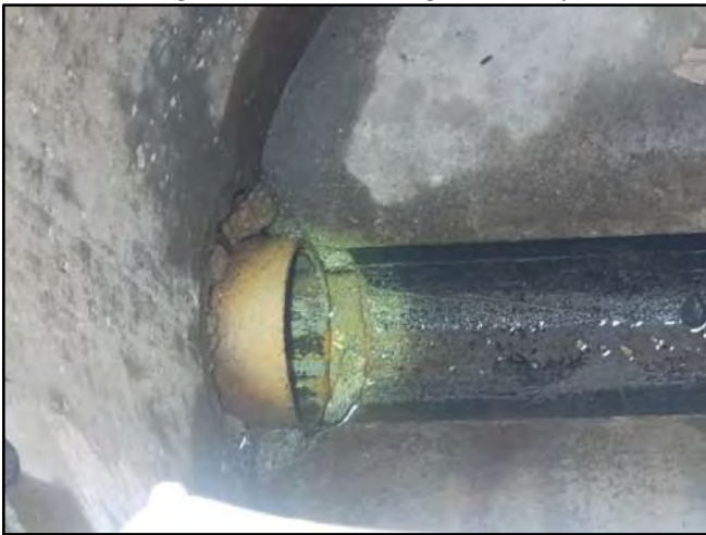
Image 5 – Missing Invert and South Effluent Connection
