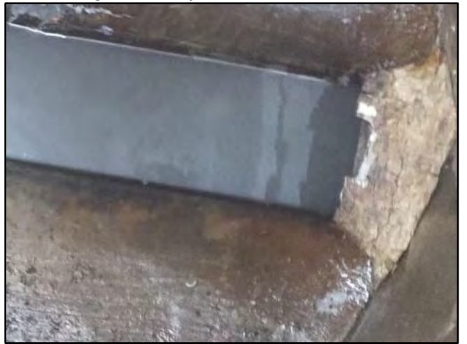
Image 6 – North Influent Connection and Dripper
