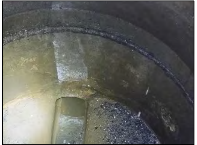
Image 4 – North Influent Connection and Spalling
