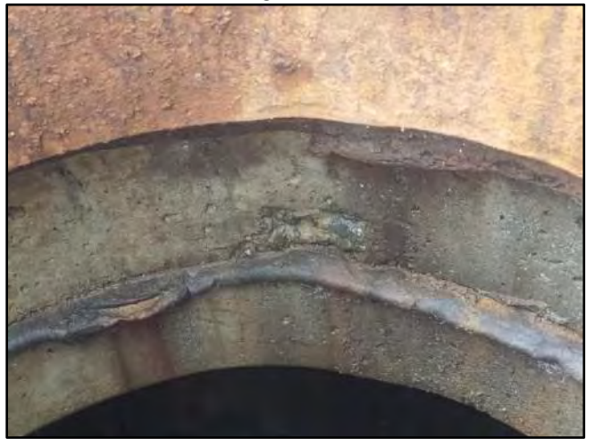
Image 6 – Chimney's Concrete Spalling
