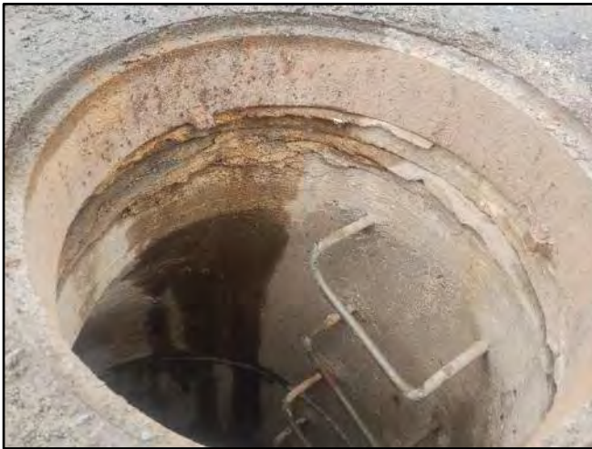
Image 3 – Cracks and Damage in Chimney
