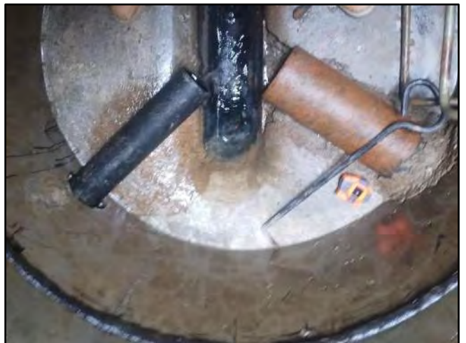
Image 6 – Elevated Pipe Connections
