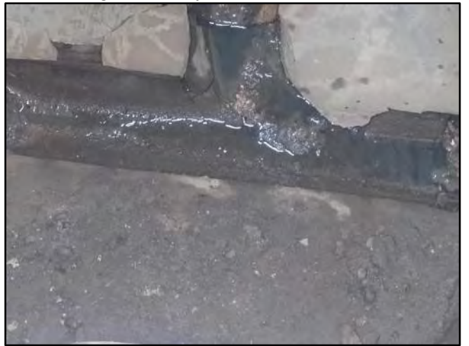
Image 6 – Missing Invert and Sediment on Shelf
