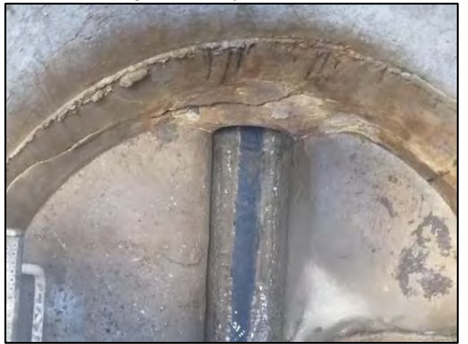
Image 6 – Base Hairline Crack
