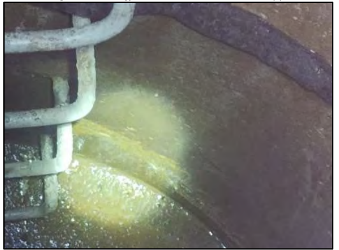
Image 6 – Missing Concrete along Base
