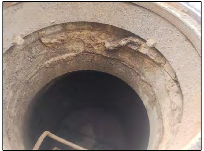
Image 6 – Chimney's Concrete Peeling
