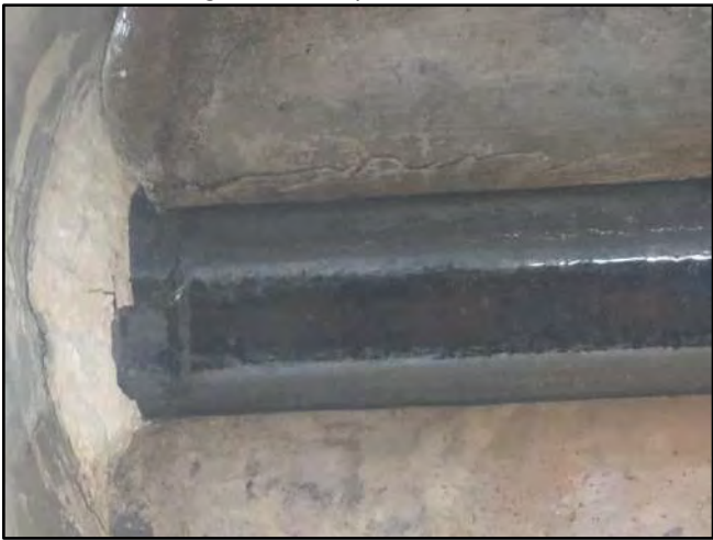
Image 5 – East Influent Connection and Crack
