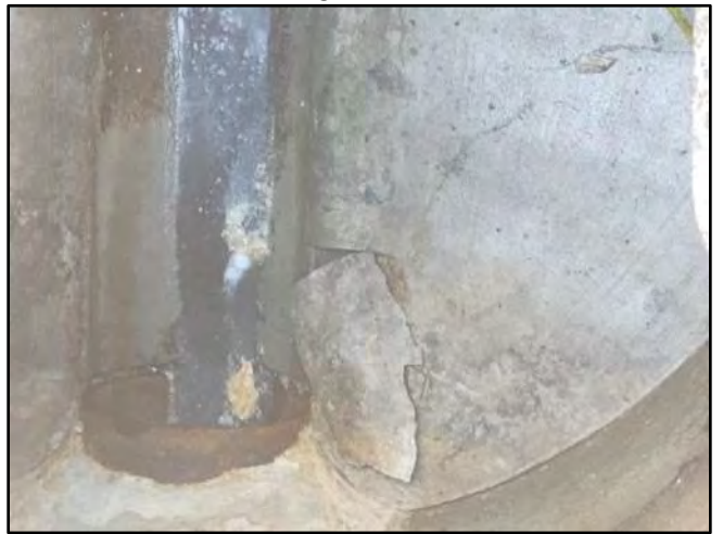
Image 6 – Fractured Concrete Section
