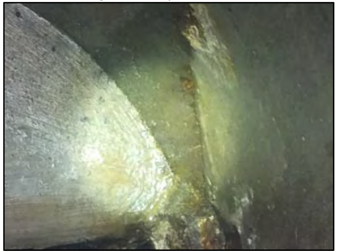
Image 6 – Crack and I&I Dripper
