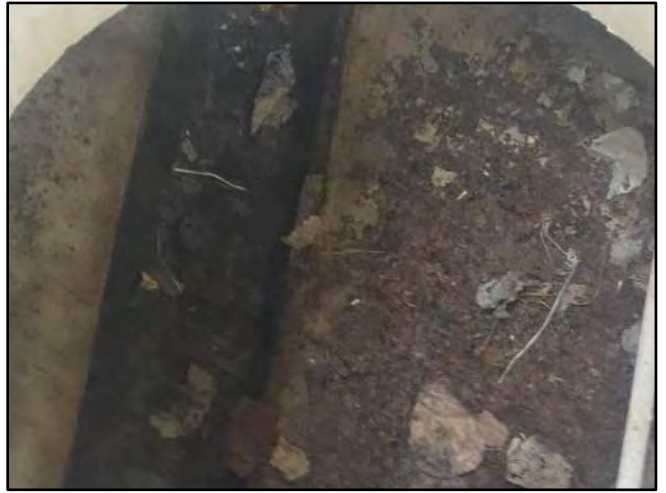
Image 4 – Debris along the Base
