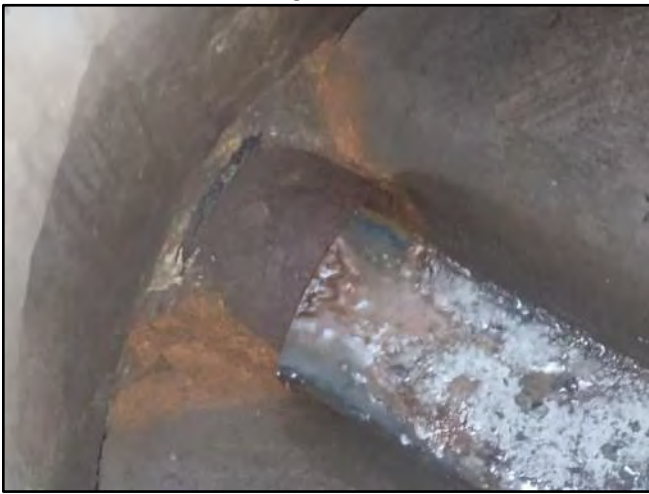
Image 5 – South Effluent Connection
