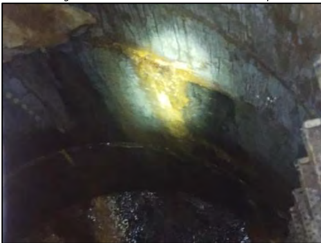
Image 5 – Crack in the Barrel
