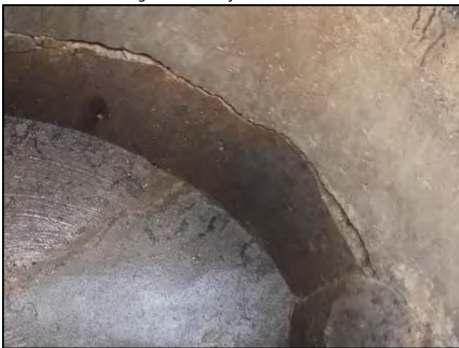
Image 5 – East side of North Crack in Base
