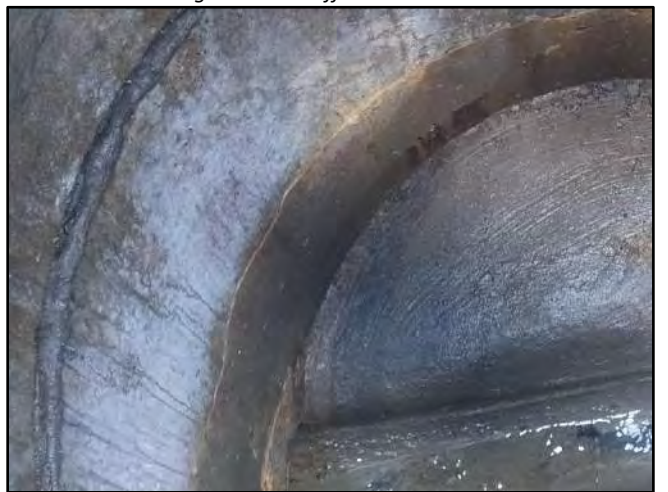
Image 6 – West side of North Crack in Base
