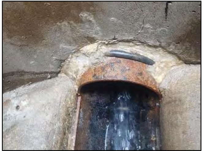
Image 4 – Effluent Connection with Exposed Gasket
