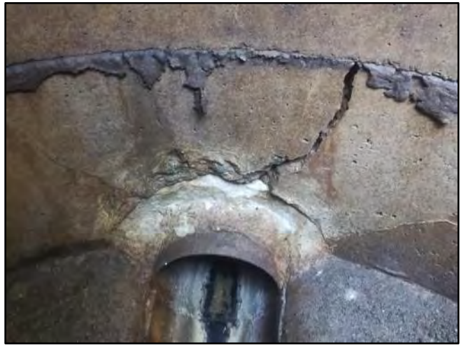
Image 4 – East Influent Connection and Crack
