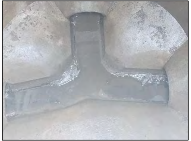
Image 4 – Standing Water in Pipes
