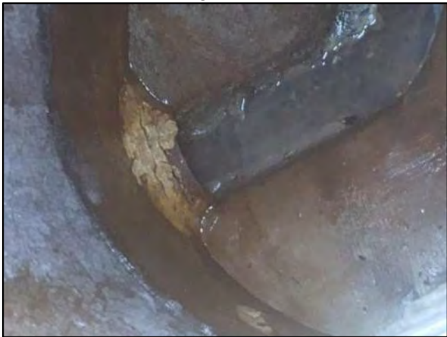
Image 5 – North Effluent Connection
