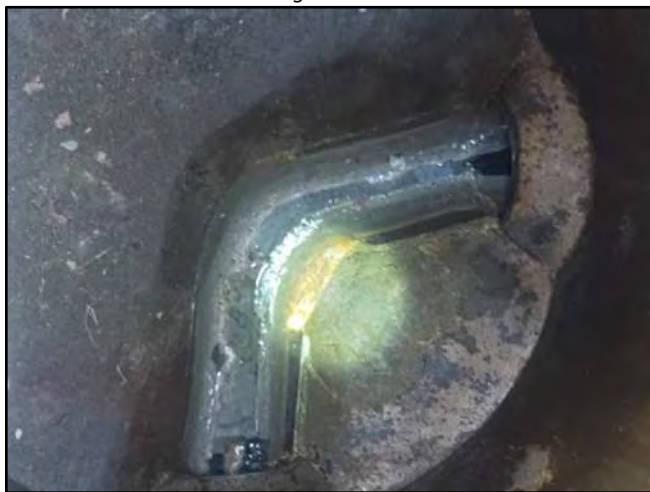
Image 5 – Missing Concrete on Shelf
