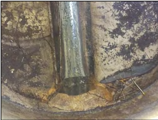
Image 3 – South Influent with Missing Invert
