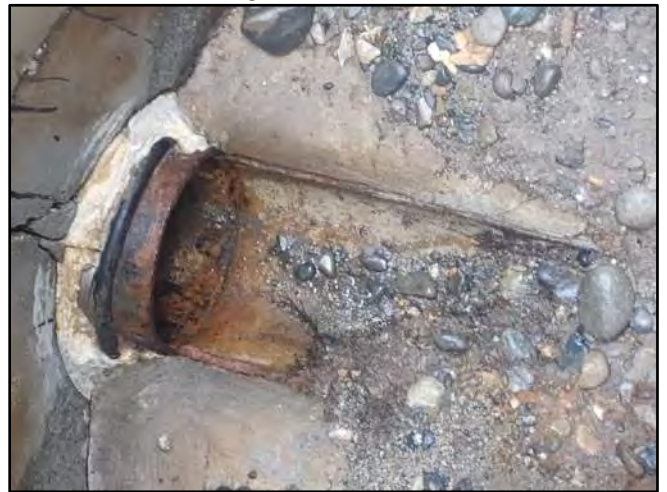
Image 6 – East Effluent Connection
