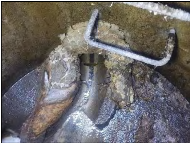
Image 5 – Deteriorating North Influent Connection
