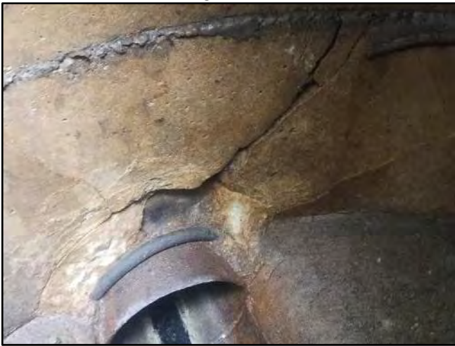
Image 5 – West Effluent Connection and Crack
