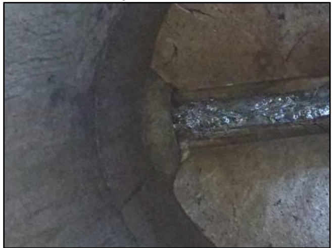
Image 6 – North Effluent Connection
