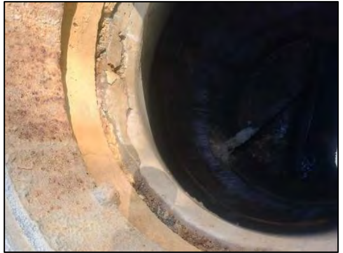
Image 2 – Cracking Along top of Cone and Joint
