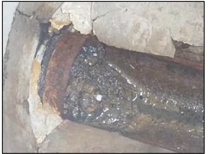
Image 4 – West Influent Connection and Crack
