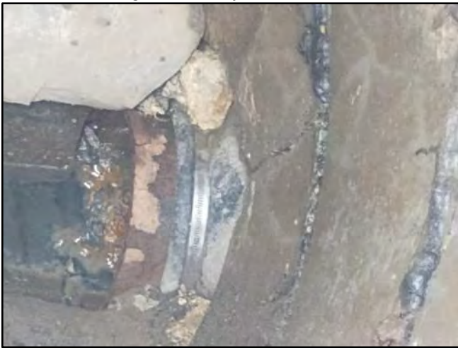
Image 5 – East Effluent Connection and Crack
