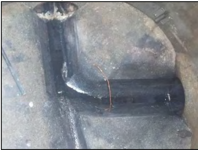
Image 5 – East Influent and North Effluent Connections
