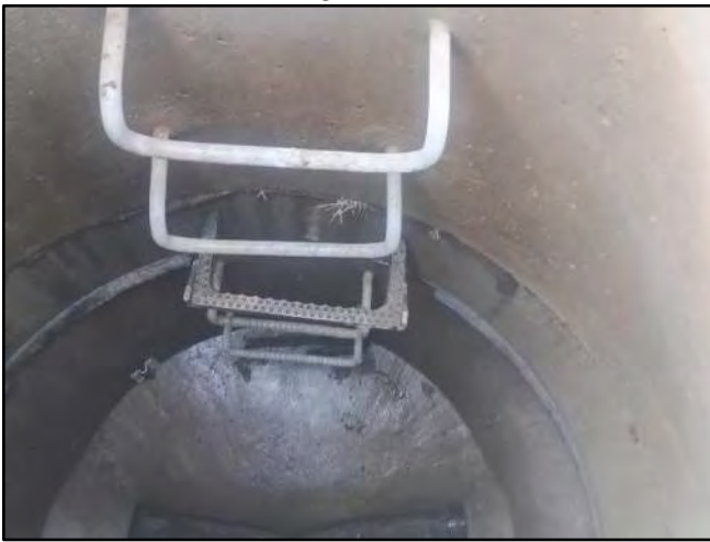
Image 5 – Minor Root Intrusion along West Section
