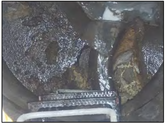
Image 4 – Missing Invert and Moisture on Shelf
