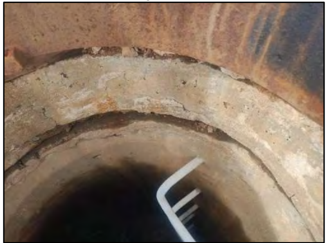
Image 6 – Chimney Sections Eroding
