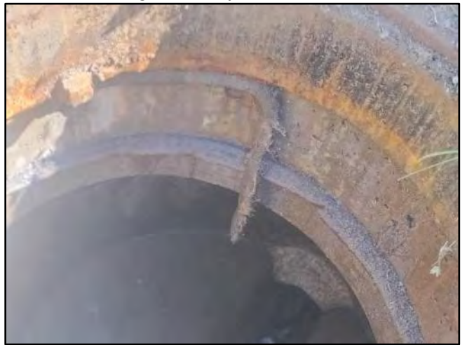
Image 6 – Sealant Between Frame and Chimney
