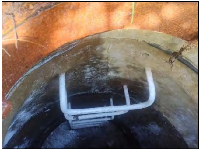
Image 6 – Crack along cone
