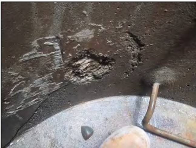
Image 5 – Missing Concrete along Base
