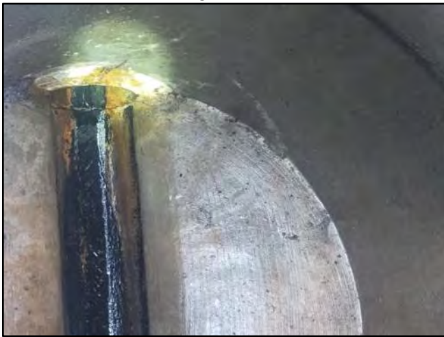
Image 5 – East Effluent Connection
