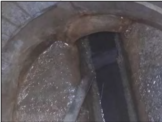
Image 5 – East Effluent Connection
