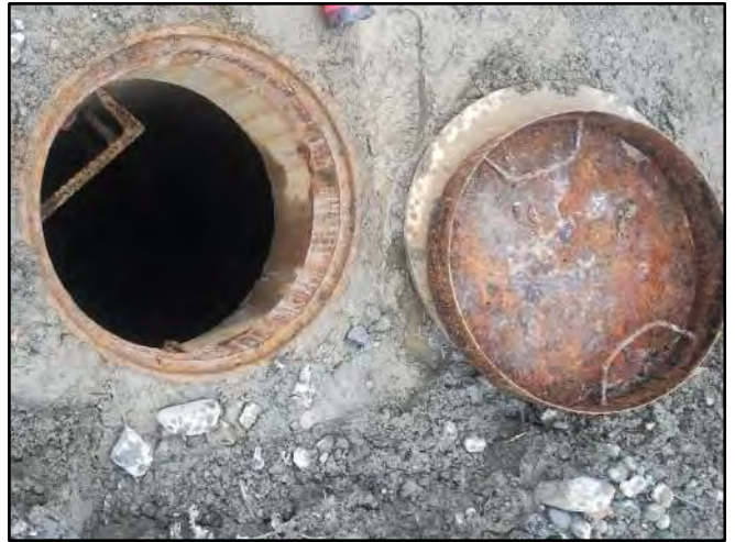
Image 2 – Frame & Unfunctional Catchpan
