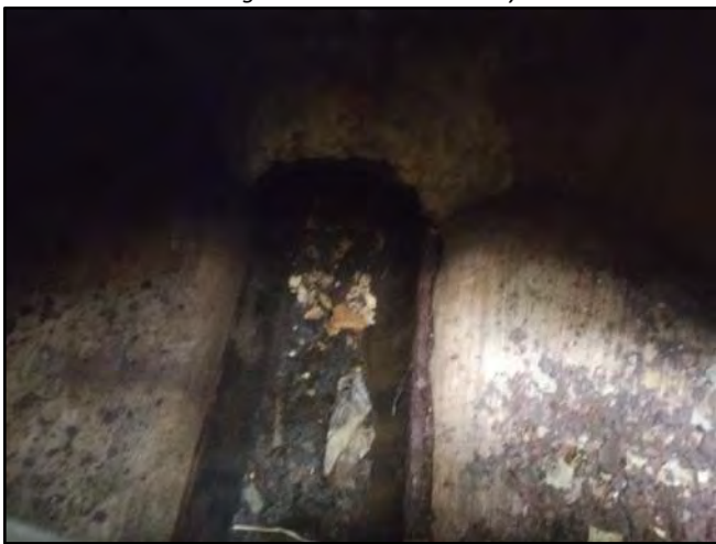
Image 5 – East Effluent Connection
