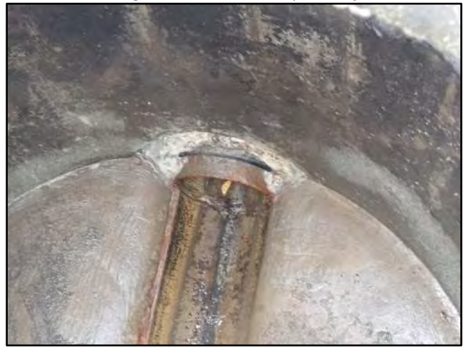
Image 6 – East Effluent Connection
