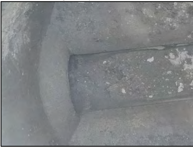
Image 5 – North Effluent Connection
