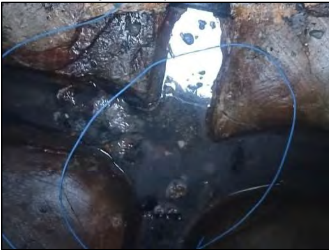
Image 5 – Missing Concrete along Shelf
