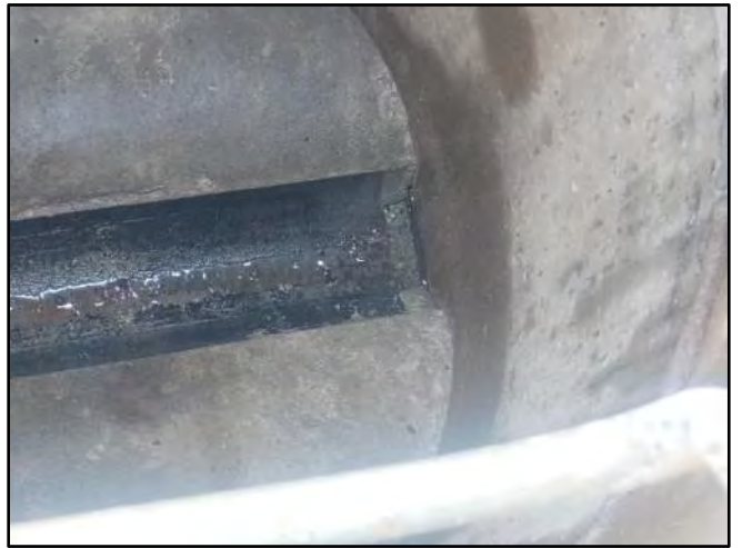
Image 4 – Missing Invert and I&I Runner
