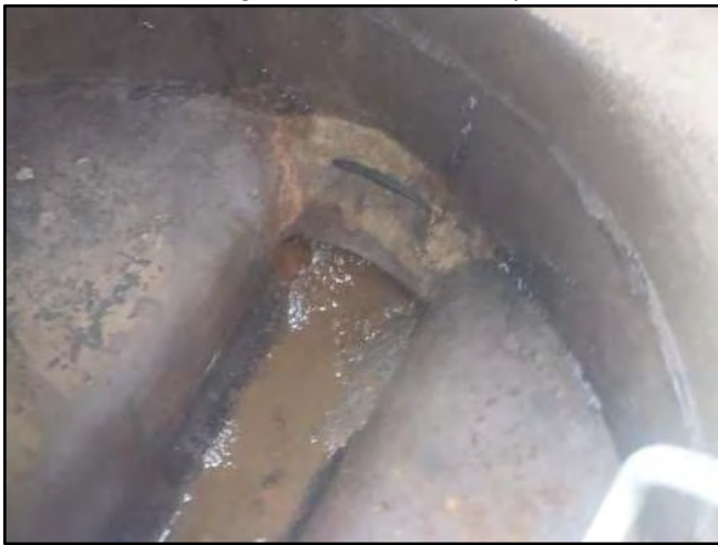
Image 5 – East Effluent Connection
