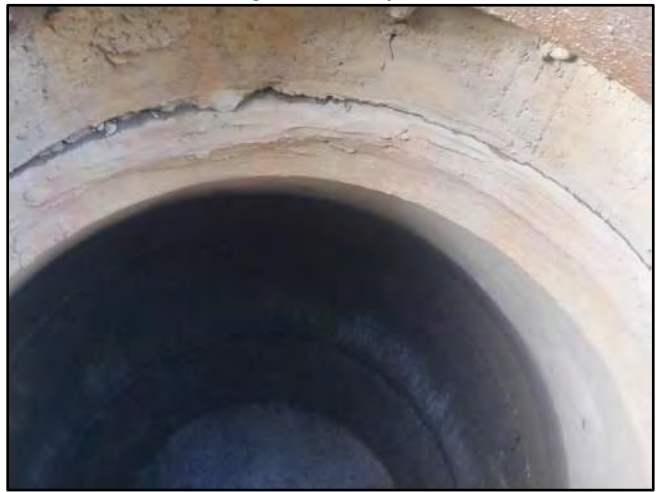
Image 6 – Missing Concrete along Chimney
