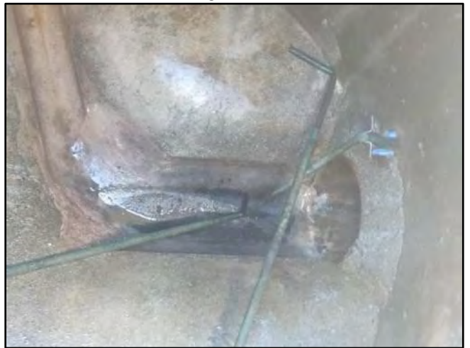
Image 6 – West Effluent and Missign Invert
