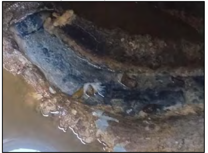
Image 6 – Solids Build-Up Lining Pipe
