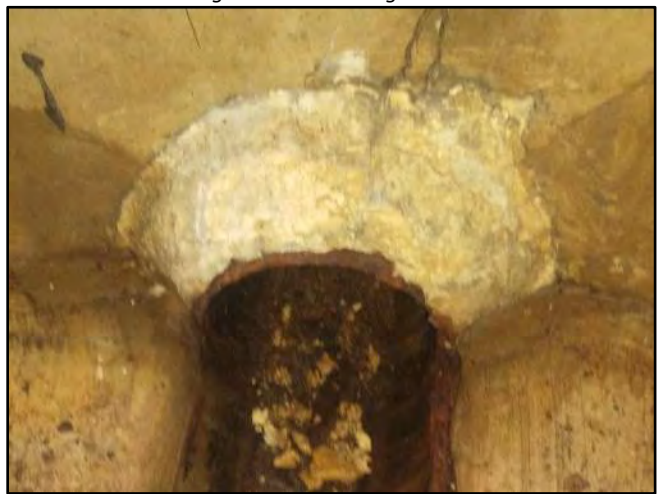
Image 6 – Cracks above Connection
