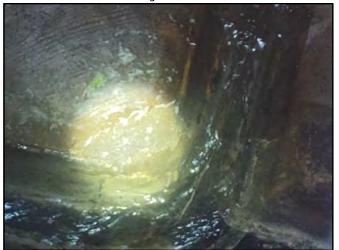
Image 6 – Missing Concrete Section
